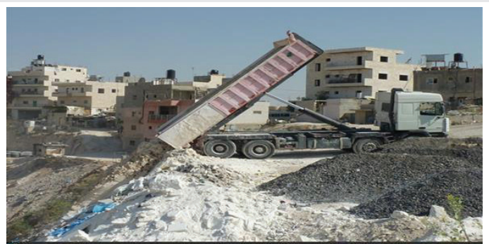
Figure 1: Stone crushing waste near residential buildings.
