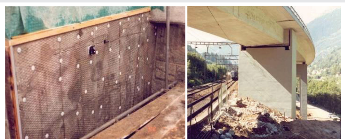
Figure 2: Titanium net fixed on the concrete of the pile with white plastic dowels (left) and restored bridge pile (right).
