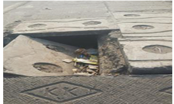
Figure 3: Condition of manhole.
