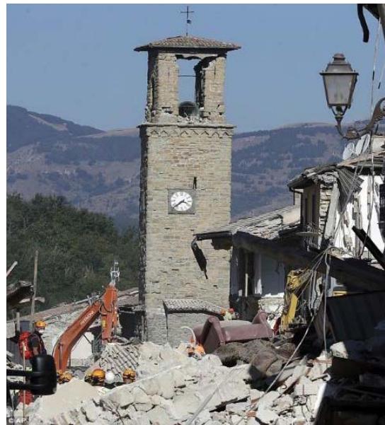
Figure 4: Church tower of 13th century standing in middle of collapsed structures.
